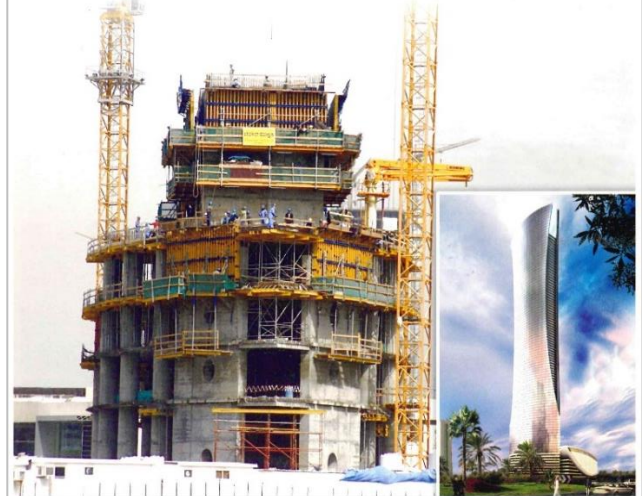
The different formwork systems supplied by Doka are in use at Qatar Navigation Tower as shown in the photo
